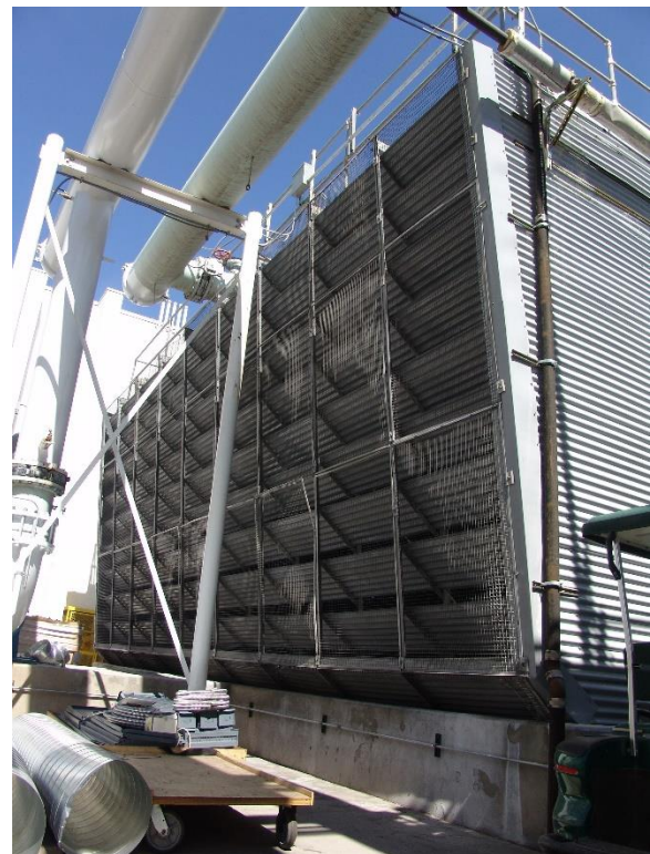
Image: Commercial cooling tower
